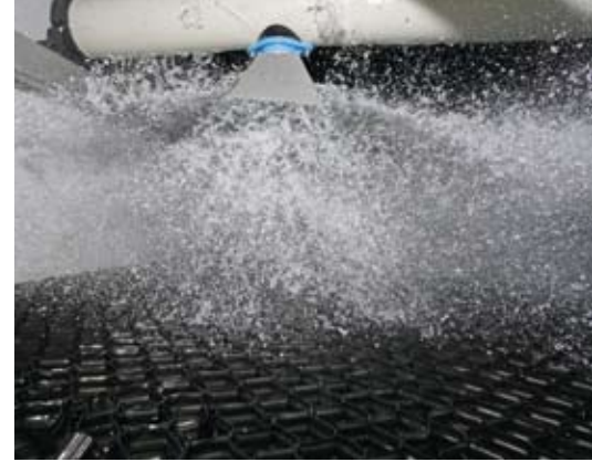
Water distribution in a cooling tower
