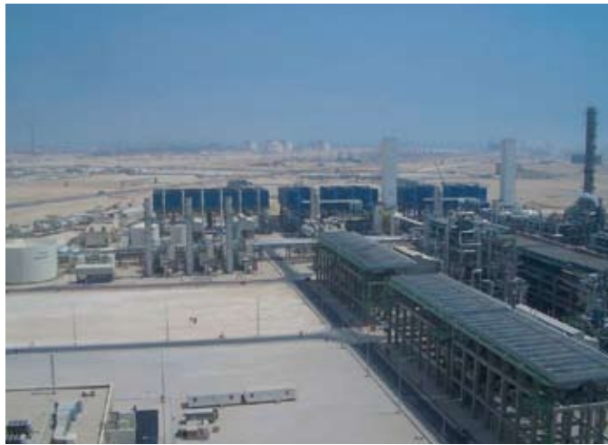
New Fuels: Air Fin Coolers and Air Cooled Condensers in a GTL plant, manufactured by Batignolles Technologies Thermiques
