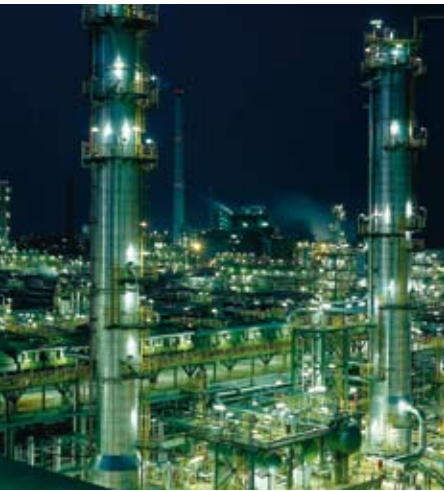
Air Fin Coolers at the Total refinery Mitteldeutschland, Germany
